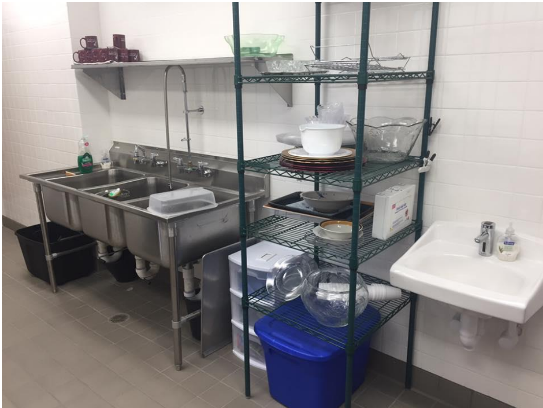
Lakewood Café Kitchen – Sinks and Storage
